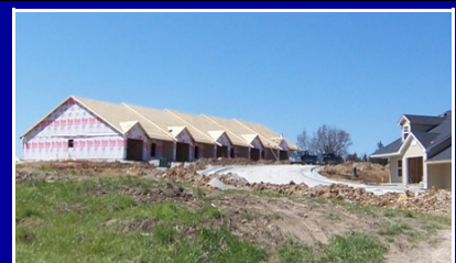
Construction of Senior Villas continues at Grayhawk Village located at Old Highway 50 and Echo Valley Road.
