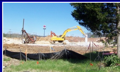
Excavation and drilling continues at site of future AutoZone, located at Hwy 50 & S. McKinley.
